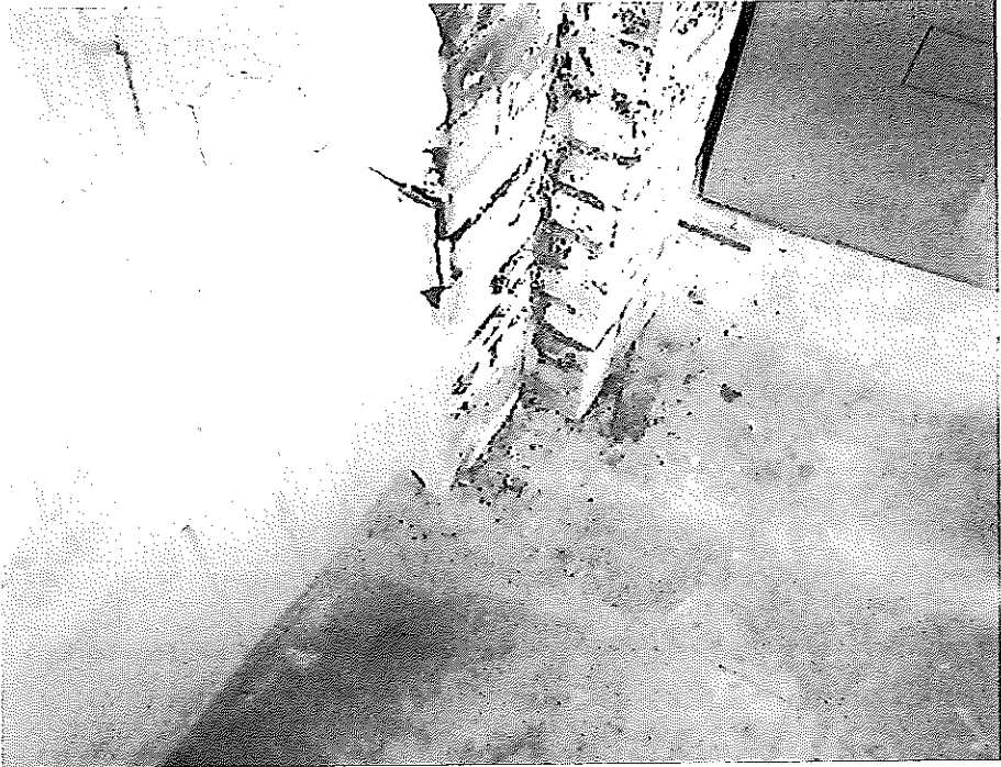
Debris and brick deterioration in the basement
