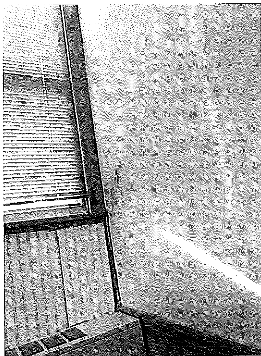
Damaged wall where moldy material had reportedly been cleaned/stripped
