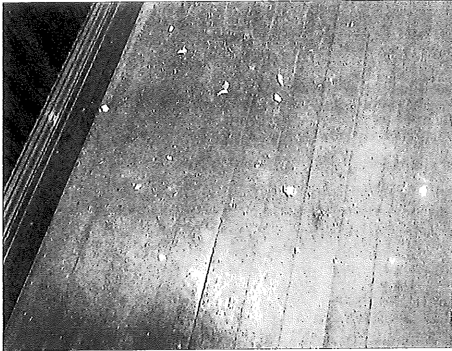
Dust and debris, including debris from foam insulation of attic floor
