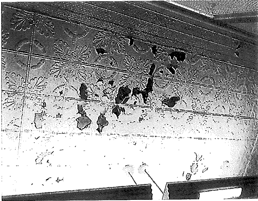
Flaking paint on upper level ceiling
