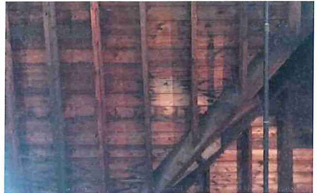
Figure 4: Water staining on the underside of the wood-plank deck and wood rafters at the roof valley.
