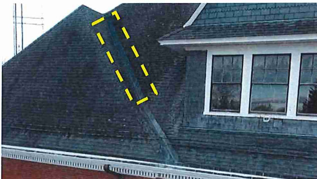
Figure 16: Drone image shows the copper valley flashing above the reported leak area at the northeast corner of the building. The flashing appears to have open seams, one that appears reverse-lapped (dashed outline) that could allow moisture to bypass the roof system.
