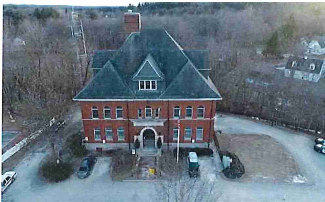
Figure 1: Drone image of the front of the Police Department roof, which consists of asphalt shingles.
