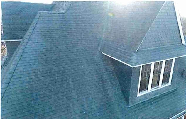
Figure 11: Drone image shows deterioration of shingles on the west side roof.
