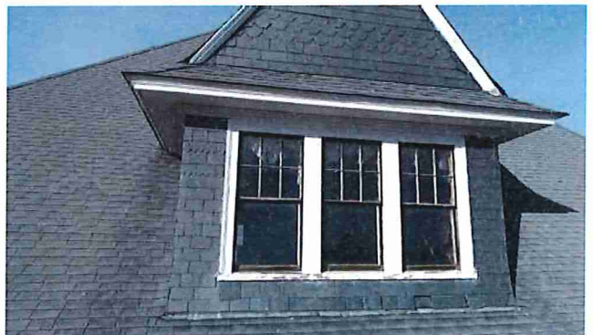
Figure 7: Closeup photo of wood windows and painted wood trim on a representative dormer.
