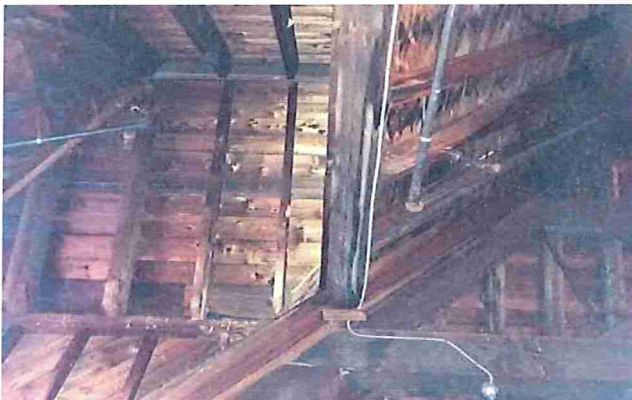
Figure 2: Water staining was noted on the underside of the wood-plank deck and on wood beams at the dormer on the west end, south side of the building.
