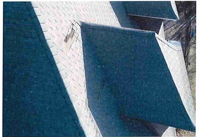
Figure 13: Drone image shows damaged and missing asphalt shingles adjacent to the southwest dormer. The damage closer to the ridge is in the proximity of the reported moisture infiltration below (figure 2).
