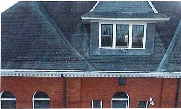
Figure 9: Drone image of the lower north side of the roof where widespread deterioration of asphalt shingles is noted.
