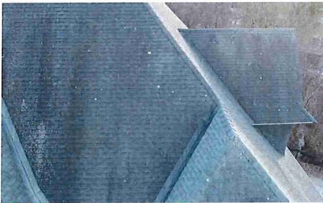
Figure 10: Drone image of the east end, north side, of the roof where widespread deterioration of asphalt shingles is noted.
