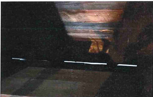
Figure 5: Photo from the building interior shows visible daylight at the roof edge beyond the wall plane. This condition provides ventilation to the attic.
