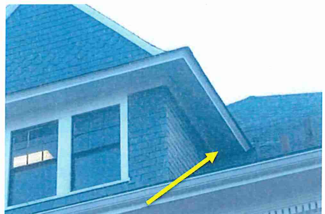
Figure 20: Deteriorated wood trim (arrow) noted on the soffit of the west-side dormer.
