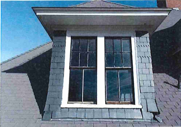
Figure 21: Closeup photo of a dormer façade shows loose, damaged and missing slate. Wood window sashes are deteriorated. Peeling paint is noted on wood trim.
