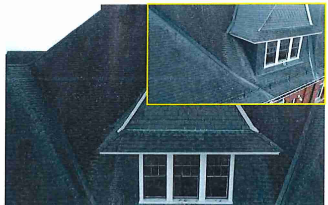
Figure 8: Drone image of the upper north side of the roof where widespread deterioration of asphalt shingles is noted.
