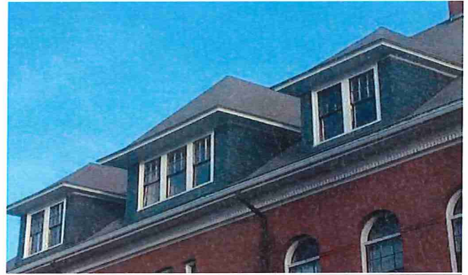
Figure 6: Dormers facades and cheek walls are clad with slate. Wood windows and painted trim accent the facades.
