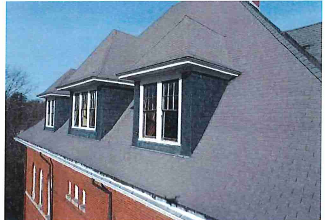
Figure 18: Drone image shows the gutter on the south edge of the roof. The gutter appears clear of debris and obstructions to the downspouts.
