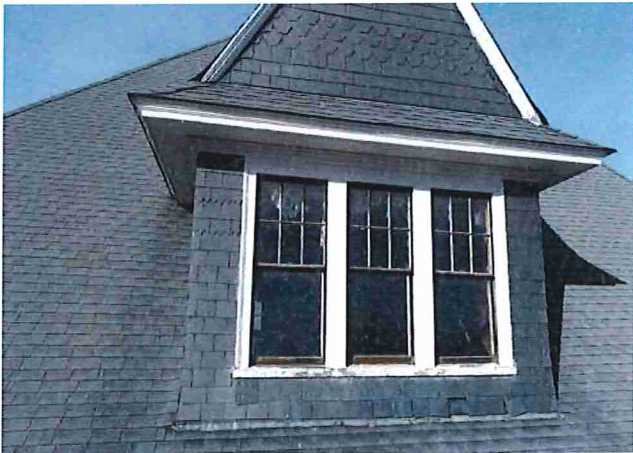
Figure 22: Closeup photo of a dormer façade shows loose and missing slate. Wood window sashes are deteriorated. Peeling paint is noted on wood trim.
