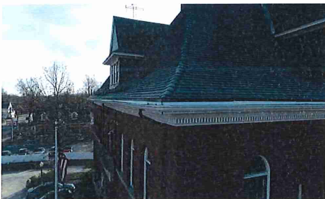
Figure 17: Drone image shows the aluminum gutter on the north and west edges of the roof exhibit some deflection. The gutter flange appears loose on the north edge of the roof. The gutter generally appears clear of debris and obstructions to the downspouts.
